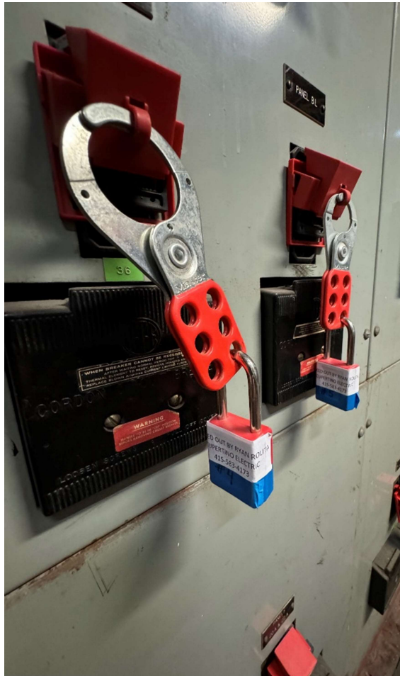
Lock-out Tag Out in place on existing switch gear
