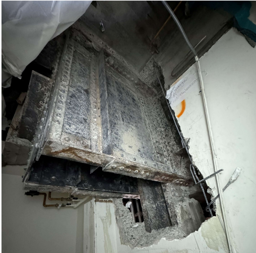
Concrete chipped to expose 65" deep steel beam
