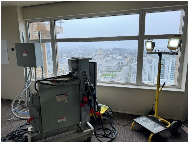
Temporary power and lighting distribution installed
