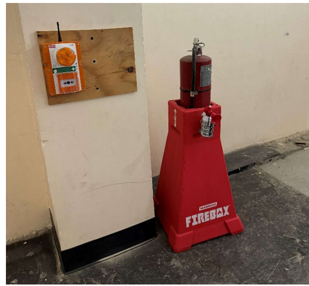
Temporary fire alarm system
